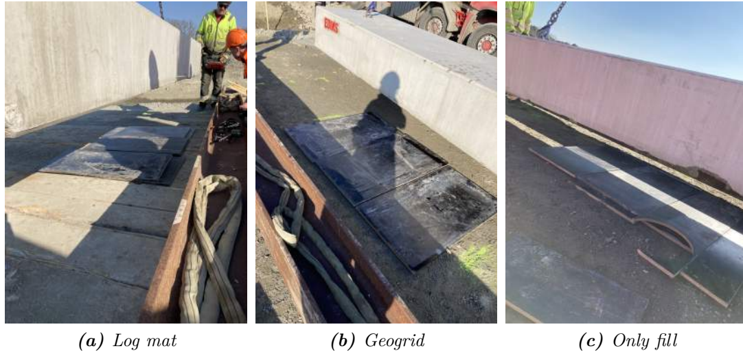
Figure 3.14: Solution with plywood boards to ensure contact of the simulated track with working platform.
